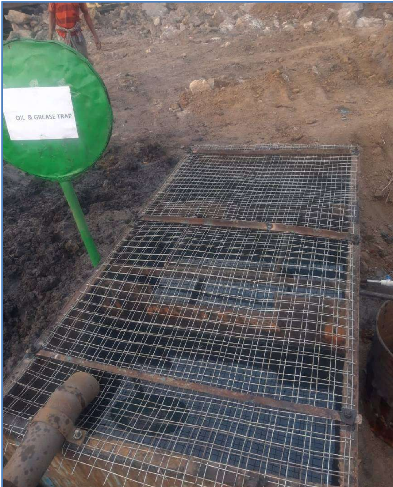
Picture 5 – Oil & Grease Trap
