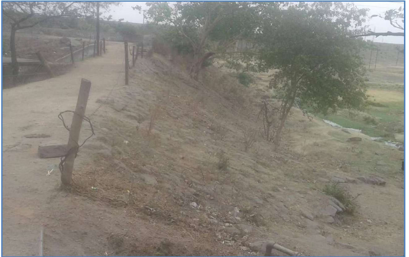
Picture 3 - Stone Pitching/embankment at Kari Jore
